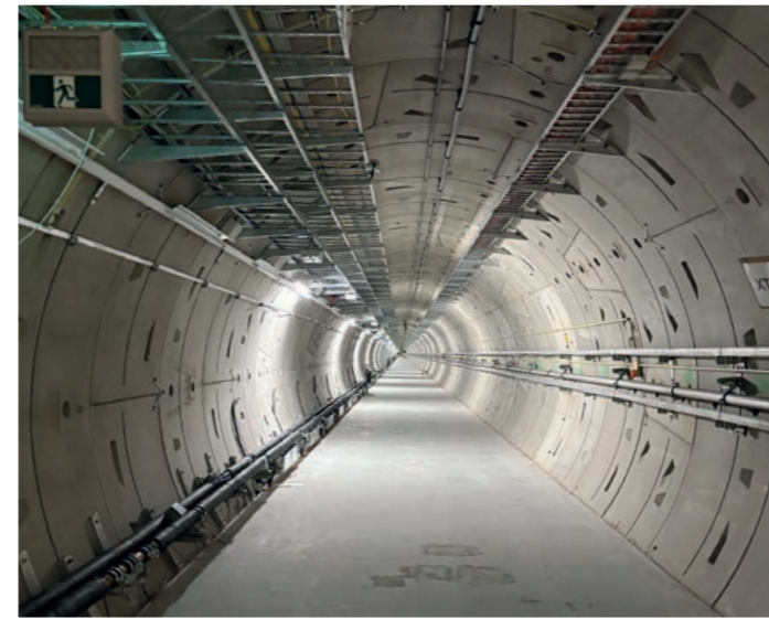
Figure 2 View into the XTD8 tunnel, in which the ELBEX beamline is to be installed
