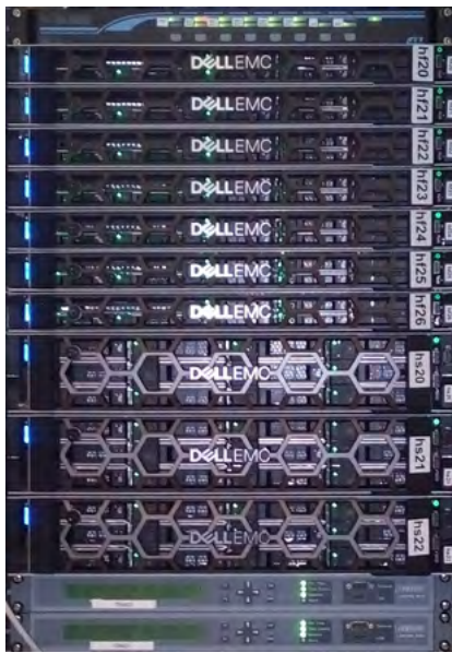
Figure 1 Front view of the new H.E.S.S. DAQ computing rack
