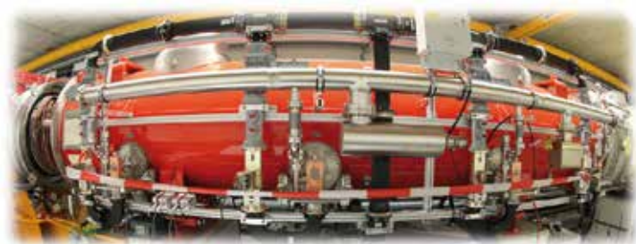
Figure 1 AH1 module in the tunnel, equipped with its RF distribution and coupler vacuum lines
