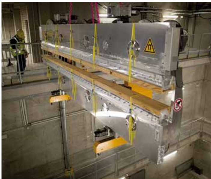
An undulator segment is lowered down a shaft into the underground tunnels of the European XFEL.
