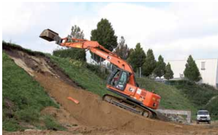
First digging at the FLASH accelerator tunnel marks the construction start for FLASH II.
