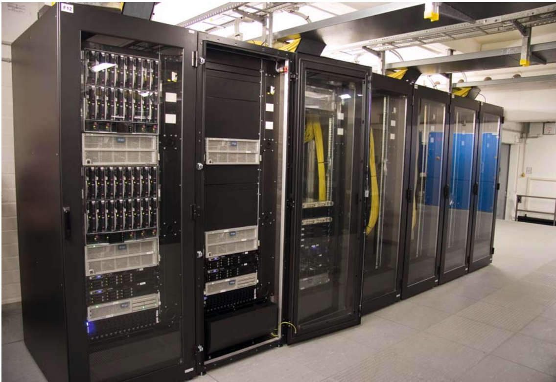
Abbildung 6: Prototyp-Installation der National Analysis Facility (NAF).
