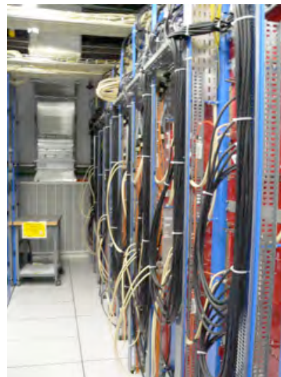
Figure 5: The front of the RCT Racks. Additional, temporary cables seen are for testing.
