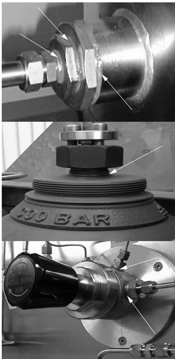
Fig. 7. Examples for applying non-outgassing epoxy (Stycast 1266 [20]) as seal for gas fittings. Arrows indicate exact locations where epoxy is applied. Note that epoxy is mainly applied within threads of connecting fittings which provides the seal. Top: adapters for pipe connection to 1.5 m 3 buffer tank (appl. press. 2.5 bar abs.); middle: CF 4 gas bottle (100 bar); bottom: CF 4 pressure regulator (100 bar on high-pressure side).
