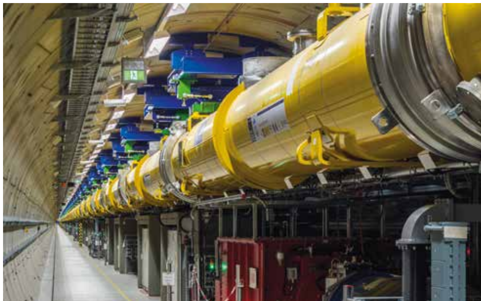
View into the 2.1-kilometre-long tunnel of the European XFEL linear accelerator. Picture: Dirk Nölle
